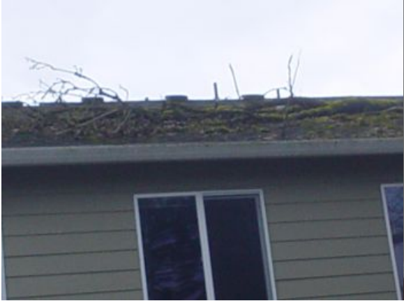
deflection note on roof,with closer inspection it appears to be cosmetic
