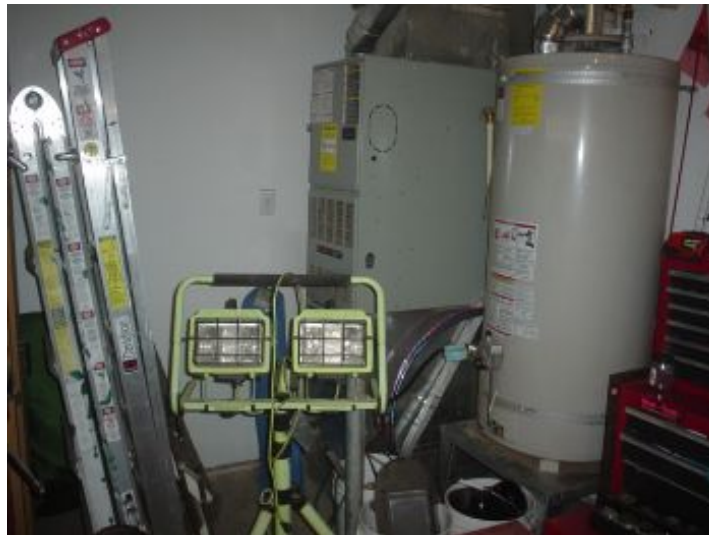
Water Heater Water Heater Condition
