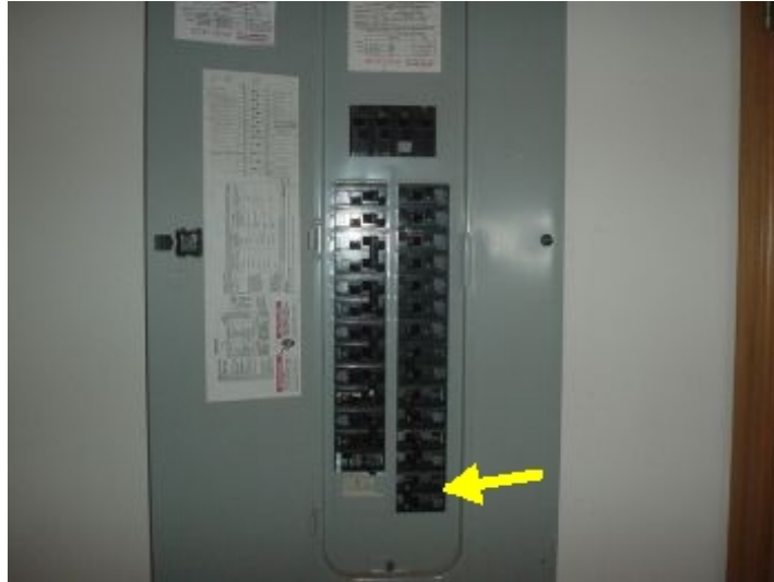
Electrical Breakers in off position
