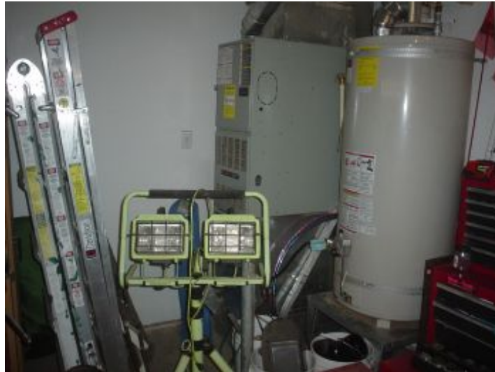
Water Heater Water Heater Condition
